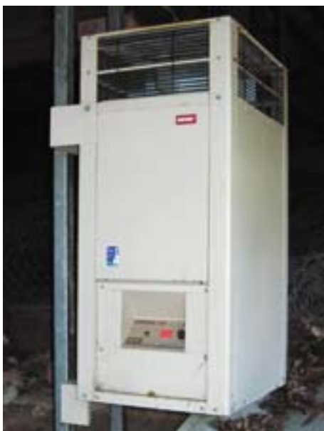
The unseen boiler that warms the hall
